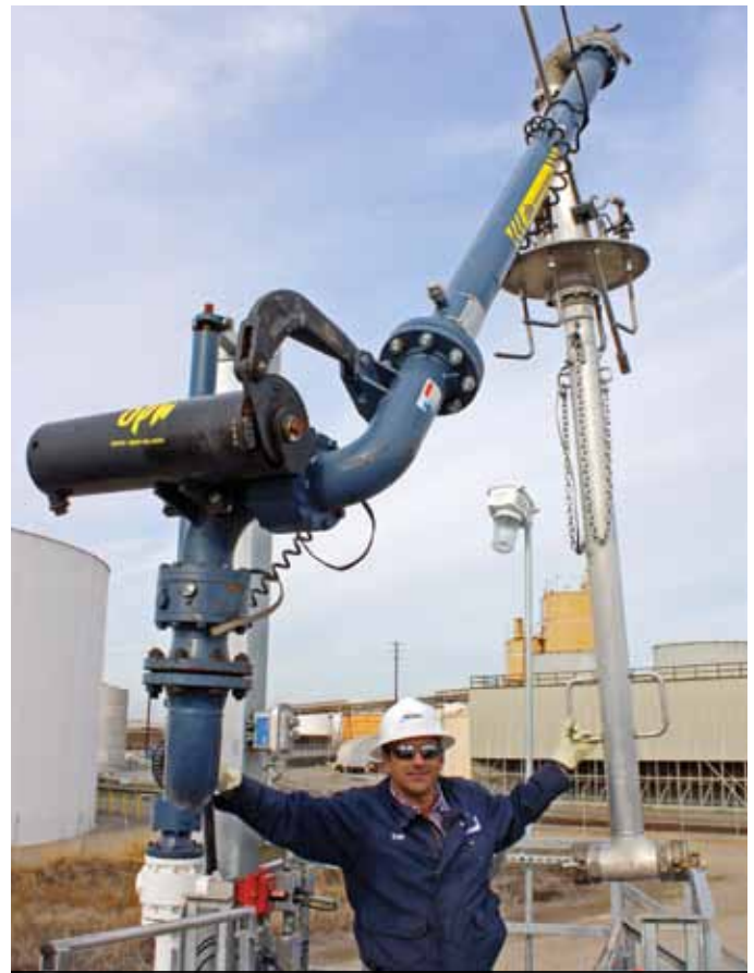
Dan Thomas, Terminal Manager at NuStar’s Stockton facility, says he can’t be more pleased with the new loading system from OPW Engineered Systems: “This really is the only way to load a railcar.”
