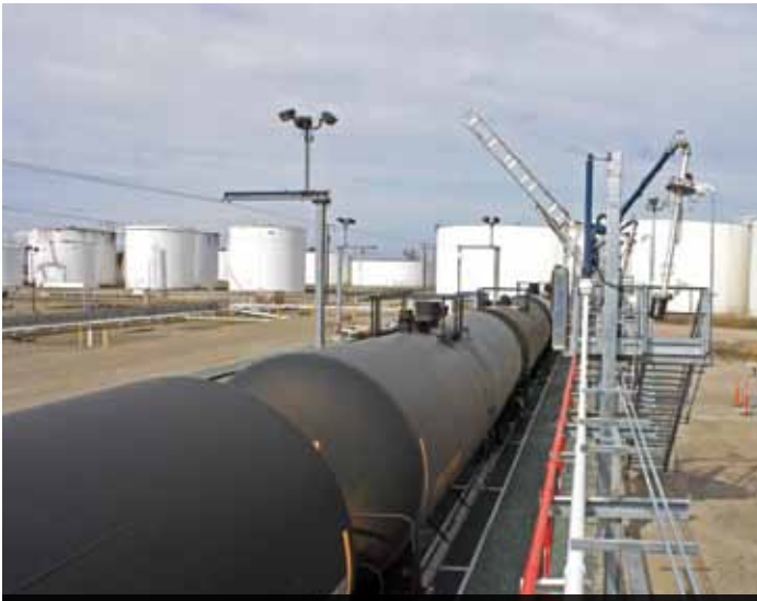
The Stockton terminal's new rail siding features six loading platforms.
